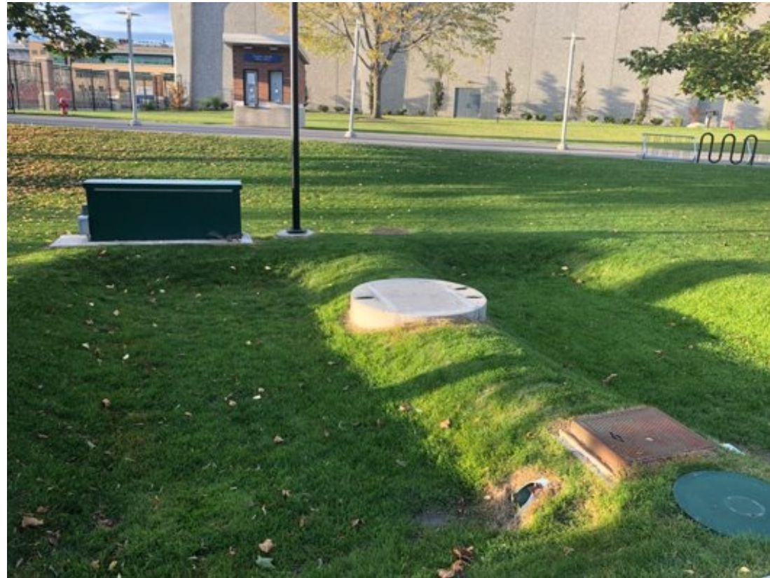
Dual-cell bioretention unit
