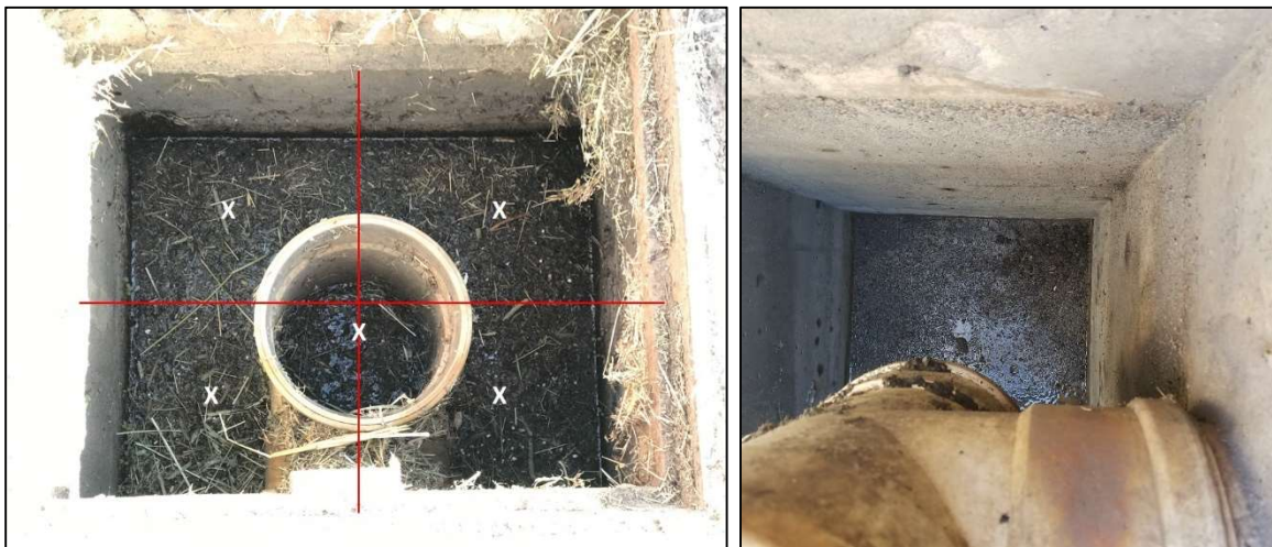
Figure 7.5 Catch basin sediment depth: measure in five locations full (left) and empty (right)
