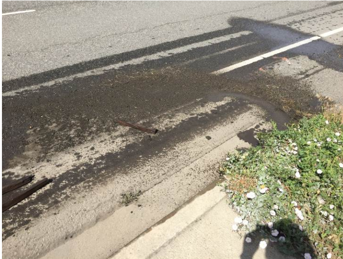
Material left behind after sweeper completed sweeping at site (just beyond crown/end of contributing basin) and lifted vacuum head below truck to drive away
