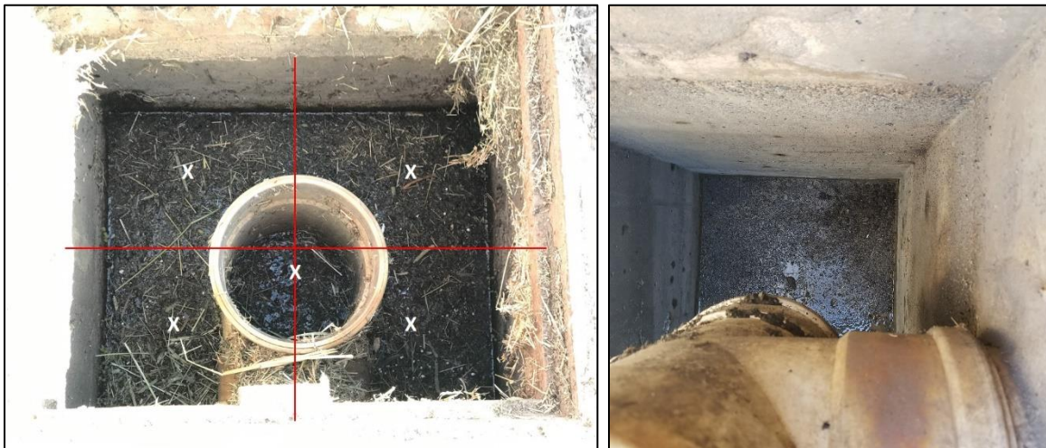
Figure 5.2 Catch basin sediment depth: measure in five locations full (left) and empty (right)
