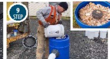
9 STEP Fill with 25-30 gallons of cleaned crushed oyster shells, about 2-3 inches below the interior overflow pipe.
