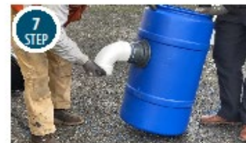
7 STEP Install 4-inch schedule 40 PVC 90-degree elbow downspout to the threaded nipple.
