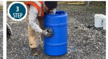
3 STEP Install 4-inch schedule 80 PVC bulkhead fitting in the hole drilled in step one.
