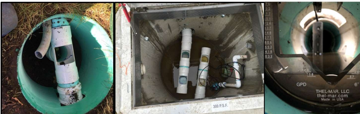
Figure 7.2 Influent sampling sump (left), manhole-effluent sampling (middle), and weir (right)
