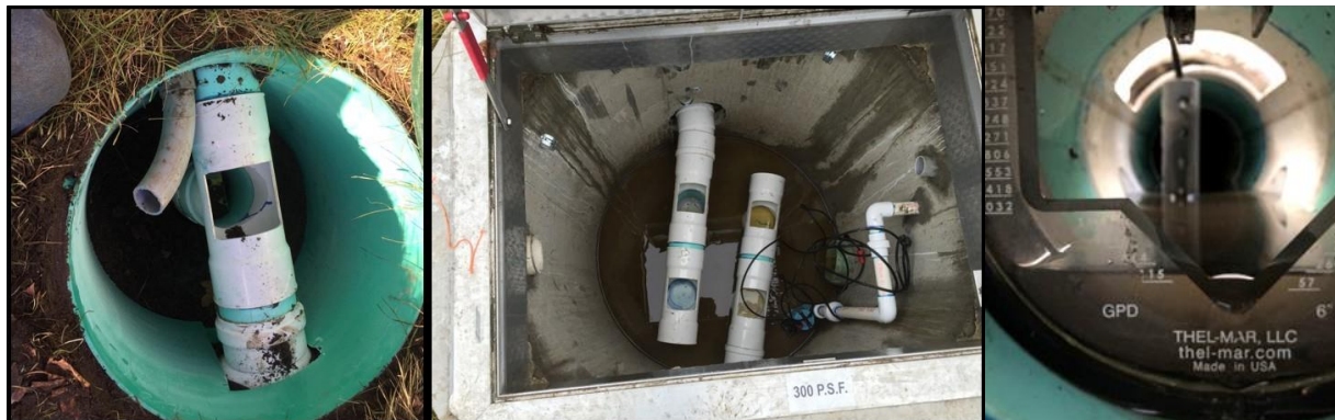
Figure 4-2 Influent sampling sump (left), manhole effluent sampling (middle), and weir (right)
