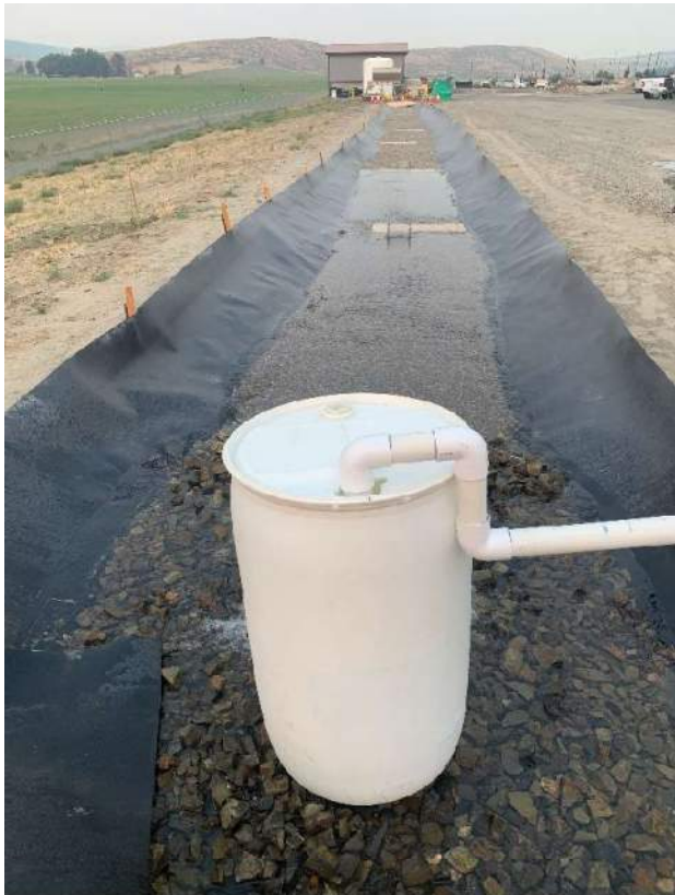
Figure D 9-15: Test of 25-year flow for Alternative 4 (sand under pea gravel) (Photo credit: Drew Woodruff, City of West Richland)
