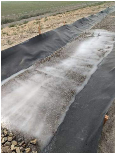
Figure D 9-7: Alternative 2 flow depth during annual load (delivered at water quality design flow rate) (Photo credit: Evergreen StormH2O)
