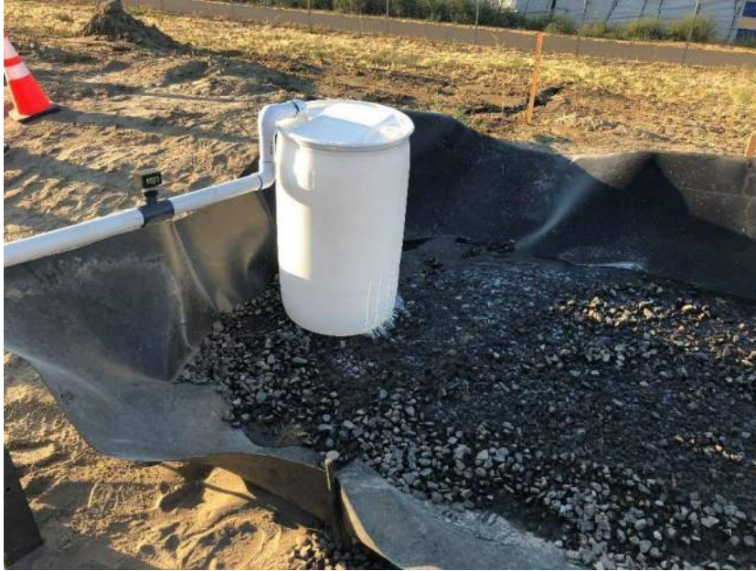
Figure 2-3. In-line flow meter and barrel used for energy dissipation (Photo credit: Brian Morgenroth, City of Walla Walla)
