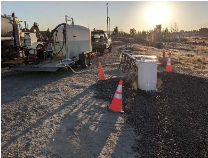
Figure 2-2. Influent distribution system during testing of final swale alternative (Photo credit: Evergreen StormH2O)
