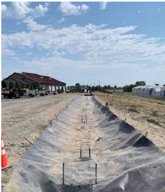
Figure D 9-3: Liner after removal of gravel and fines present below HMA gravel (Photo credit: Drew Woodruff, City of West Richland)
