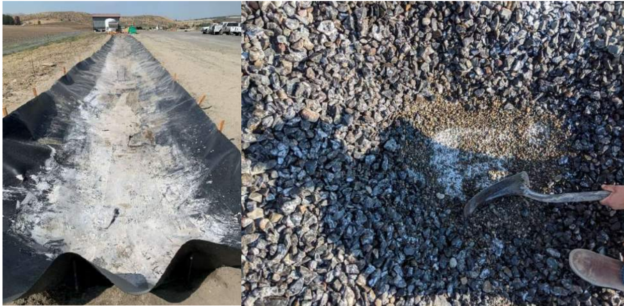
Figure 4-18. Left: Settled Sil-Co-Sil® at influent of test swale (photo from initial testing); and Right: Settled Sil-Co-Sil® in pea gravel and gravel backfill for drywells at influent (Left and right photo credit: Drew Woodruff, City of West Richland)
