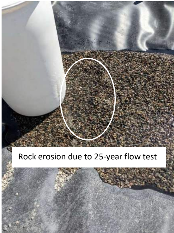
Figure D 9-4: HMA gravel erosion from 25-year flow test (Photo credit: Evergreen StormH2O)
