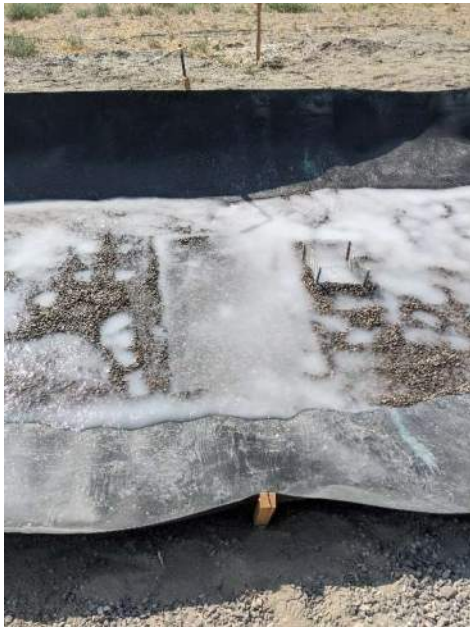
Figure D 9-9: Example of footprints and board print in pea gravel (Photo credit: Evergreen StormH2O)
