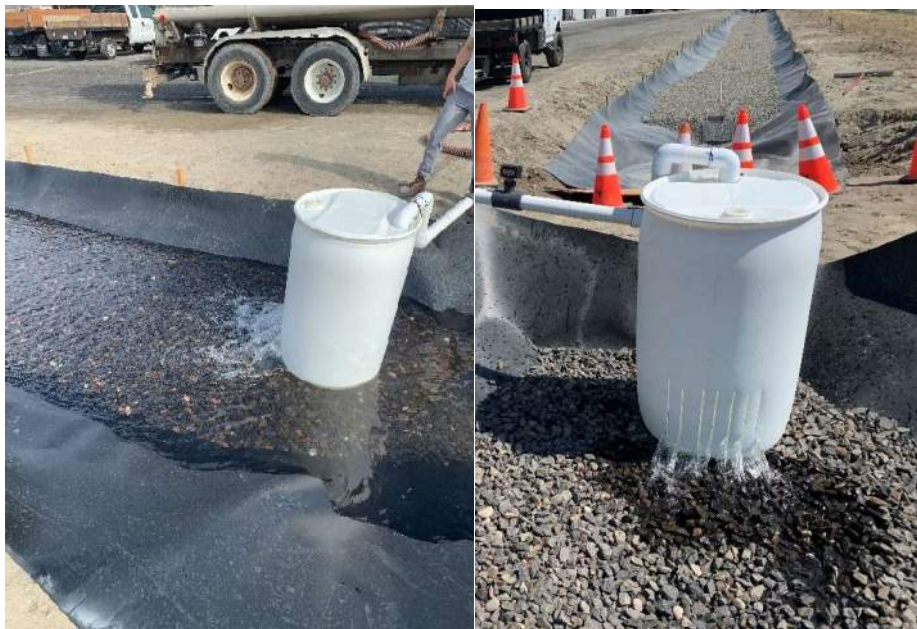
Figure D 9-11: Alternative 3 (gravel backfill for drywells) 25-year flow test (Photo credit: Drew Woodruff, City of West Richland)
