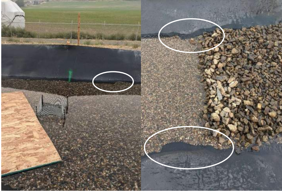
Figure D 9-8: Observations of eroded pea gravel following 25-year flow test (Photo credit: Evergreen StormH2O)
