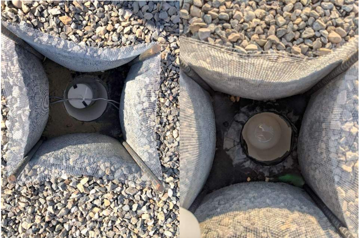
Figure 2-4. Empty sample port (left) and sample port containing grab sampler (right) (Left photo credit: Evergreen StormH2O — Right photo credit: Brian Morgenroth, City of Walla Walla)
